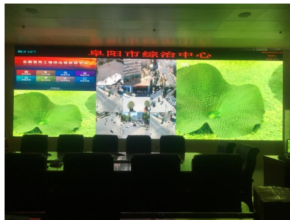
H1.25 meeting video wall in public security center in Fuyang, An' hui Province
